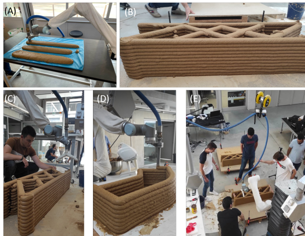
FIGURE 1 – Impression de cordons; Impression finale double buse; Impression double et simple buse
